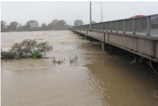
Figure 3-7 - Flooding at Buller Bridge (Stuff, 2012)
